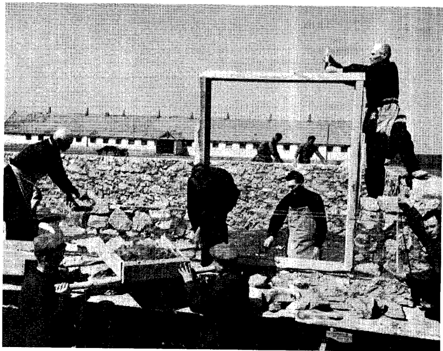
BUILDING A CATTLE BARN. A brigade of workers erecting walls for the structure on the Pobeda Collective Farm.
