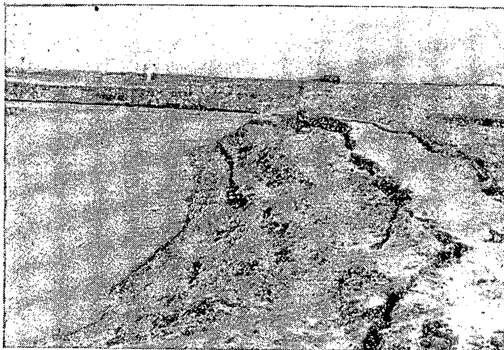
Fig. 11. Cracks in settling loess soils as a result of wetting.
