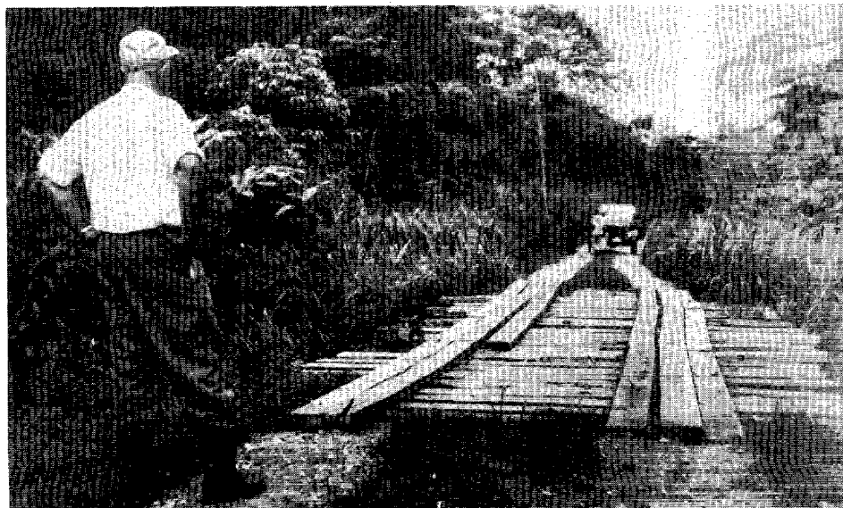
Figure 51. Road bridge in central Sumatra. This bridge has a small capacity and is unsafe for large vehicles. Note the dense vegetation along the roadway.
