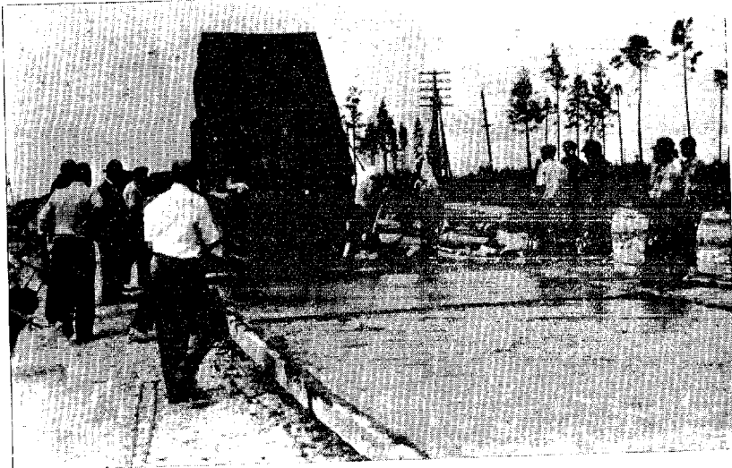
Road Under Construction at Bratsk. Wooden forms and crude screen are used; the concrete mix is delivered in an open truck; soil compaction is being performed only 300 feet in advance of the concrete.
