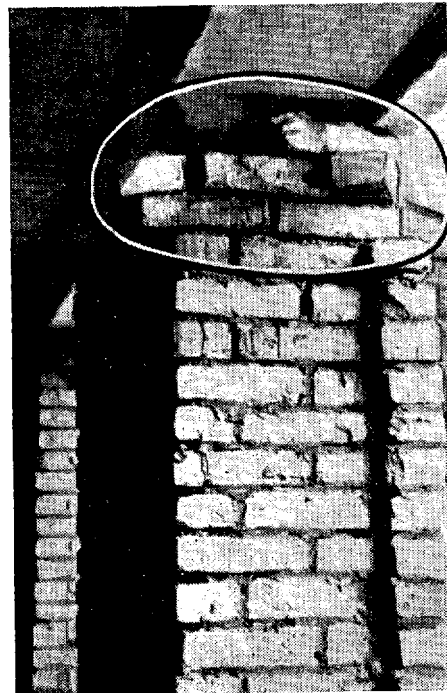
Careless bricklaying in a first-floor pillar at the Odessa failure
