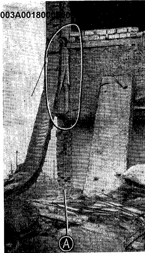
The absence of a tie-in of the cross wall to the outside wall at the Odessa failure
