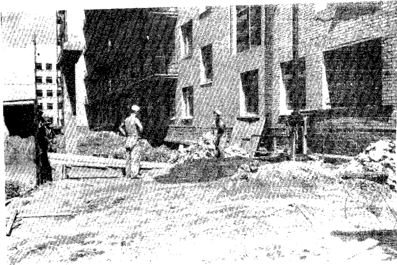
Cancer Research Center Under Construction at Leningrad. Mortar joints are not filled and pointed, thus allowing moisture to collect between the bricks where the freeze-thaw cycle will cause damage to the exterior wall. Note also the large batch of mortar dumped on the ground and the piles of rejected bricks -- further evidence of shoddy workmanship and sloppy housekeeping.
