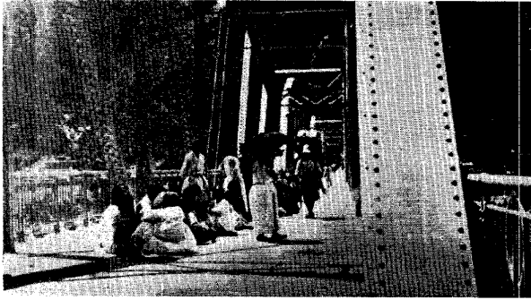
FIGURE VII - 25. Bridge over Pukban-gang (Kita-Kankō) just west of Ch'unch'on (Shunsen). Old style steel bridge.
