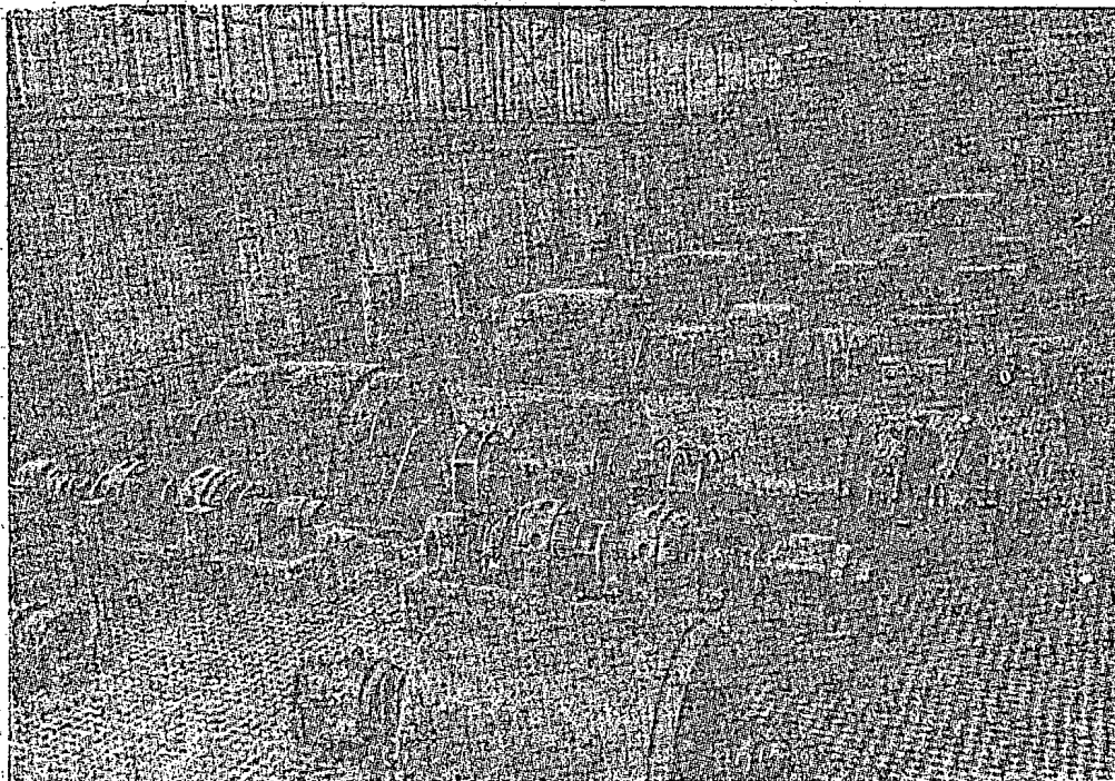
Fig. 3. General view of the synchronous-machine room.
