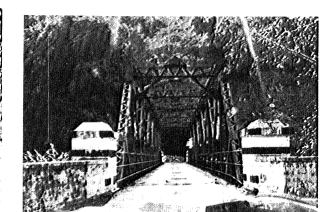
Figure 4 Three-lane road bridge on LOC Route II over Trishuli River, Nepal, 1963 (U)
