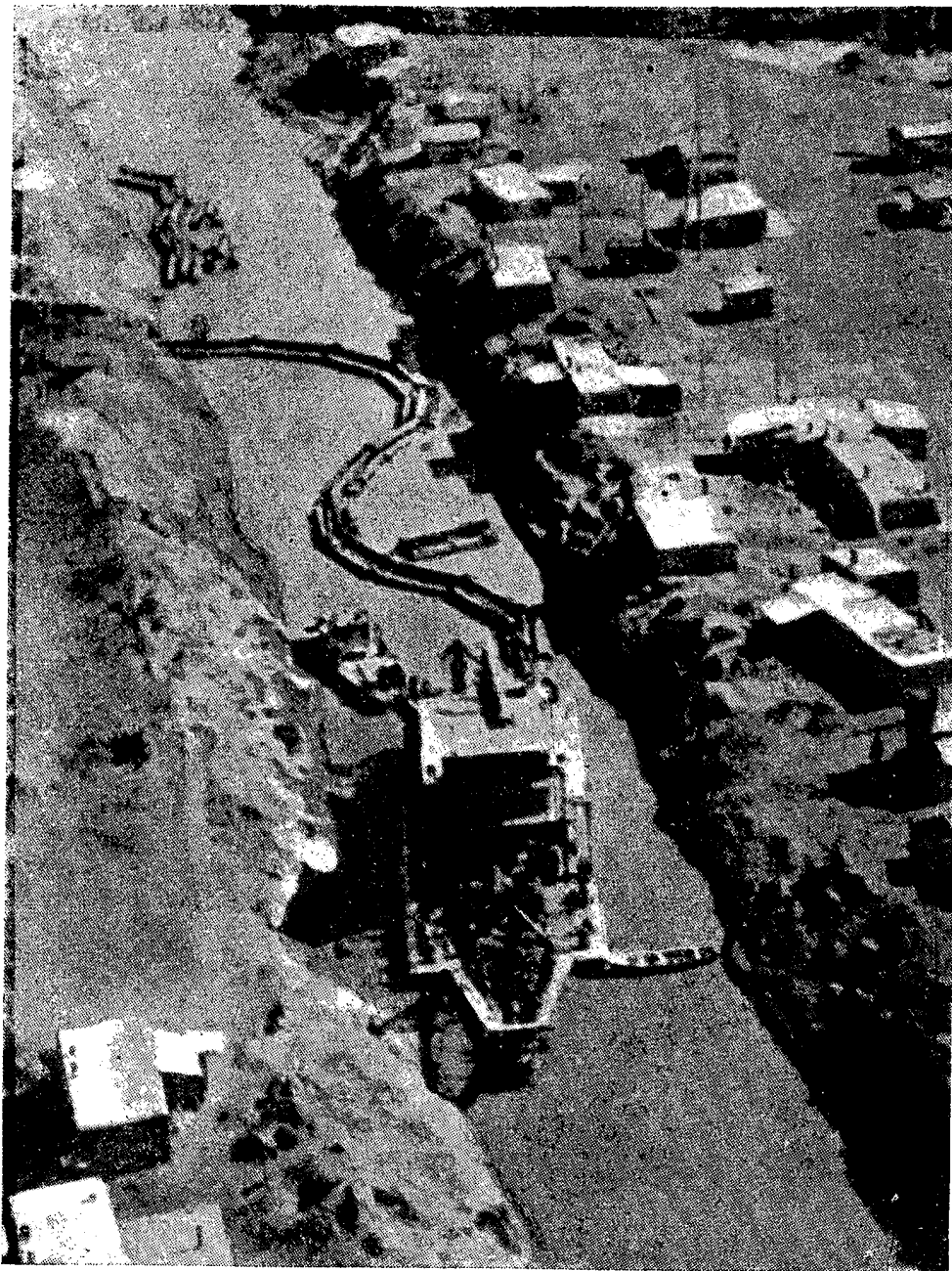
This preliminary by-pass canal has been completed; in the area where the Main Turkmenian Canal will begin
