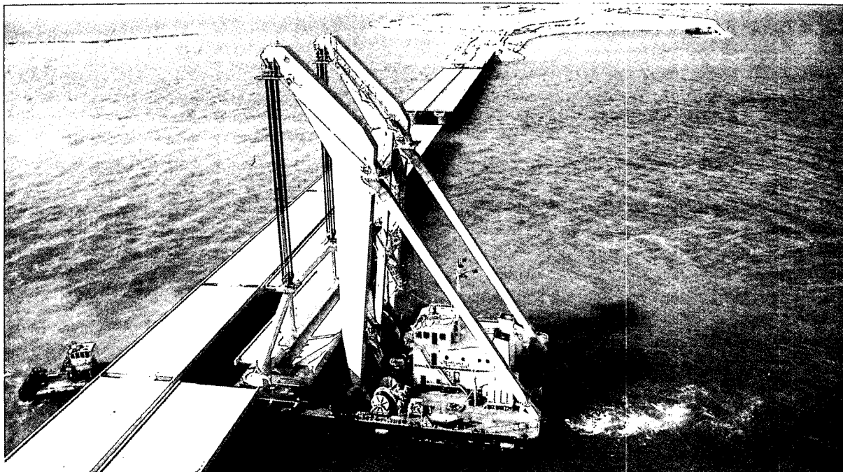
A hydraulic engineering project—all work is carried out in the open sea.
